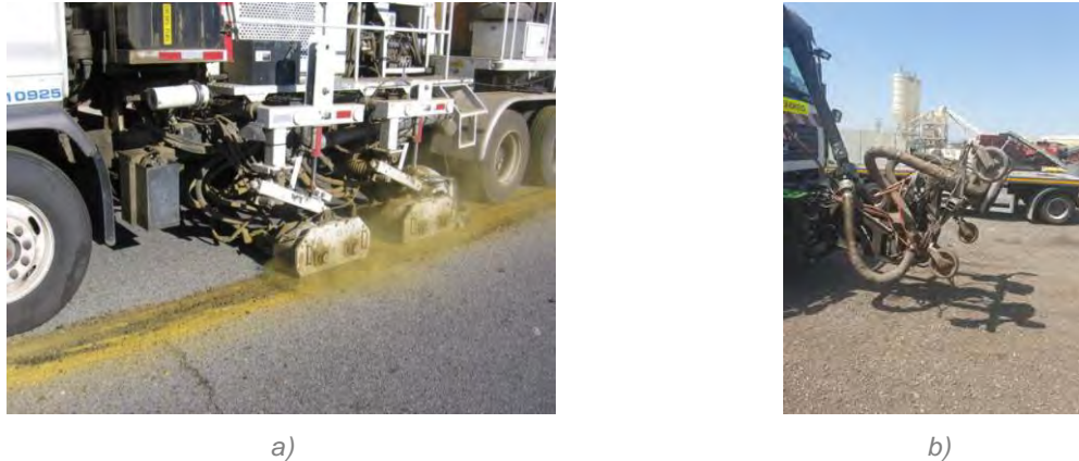
Figure 21. Different methods for the removal of markings: a) Grinding [1] and b) water-jet (PAVASAL)
